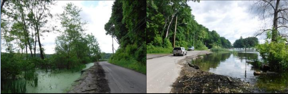
Debris and sediment on the road after 2017 flooding. Notice how close the water is to the road, with little soil left.
