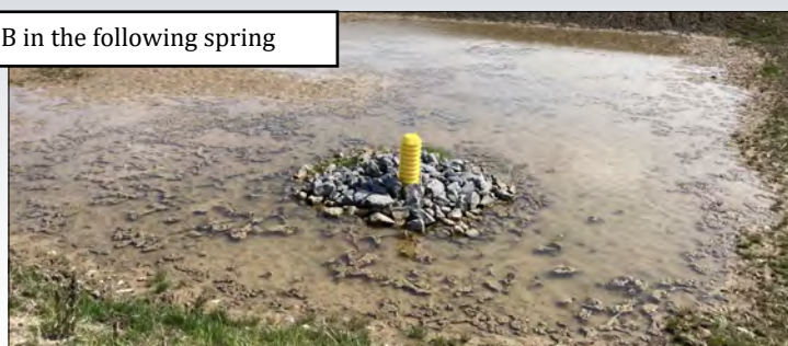
Drain section of the WASCOB with inlet riser pipe pictured
