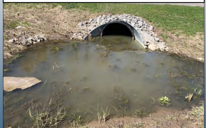
Road culvert not draining properly
